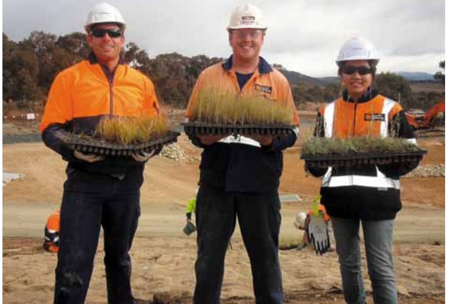
Ricky Bridge, Mathew Perkins and Winnie Ly planting native seedlings at the Williamsdale substation project.
